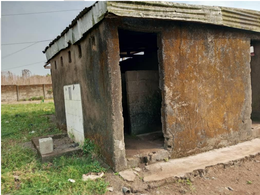
Full, dilapidated, and abandoned toilets.
