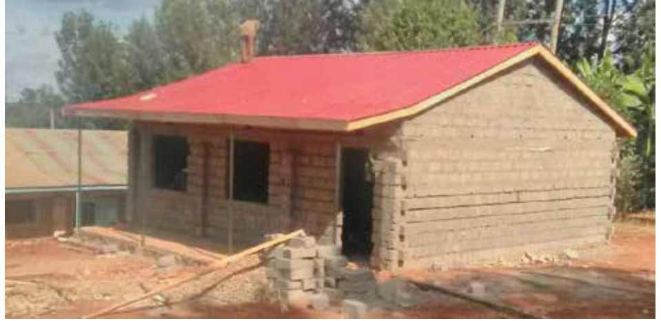
The school after. This project was funded by Los Altos Hills residents.
