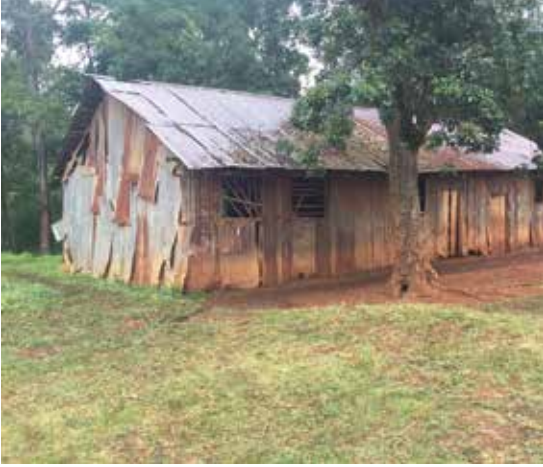
A Kenyan school before ODFL renovated it.
